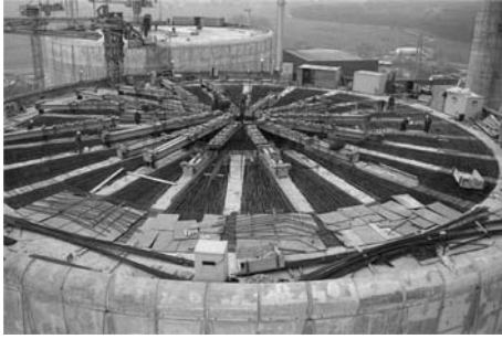
Fig. 4.5 Gundremmingen B and C reactor building roof structure, with precast wedge-shaped laid precast segments with cast concrete added locally [17]
