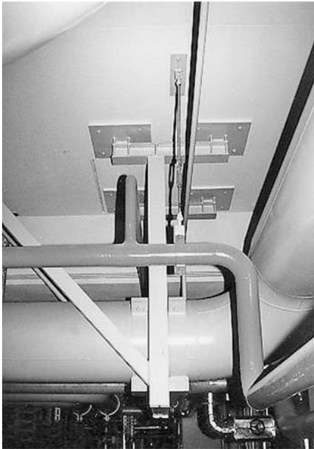
Fig. 7.4 Typical anchor plates fixed in a power plant [71]
